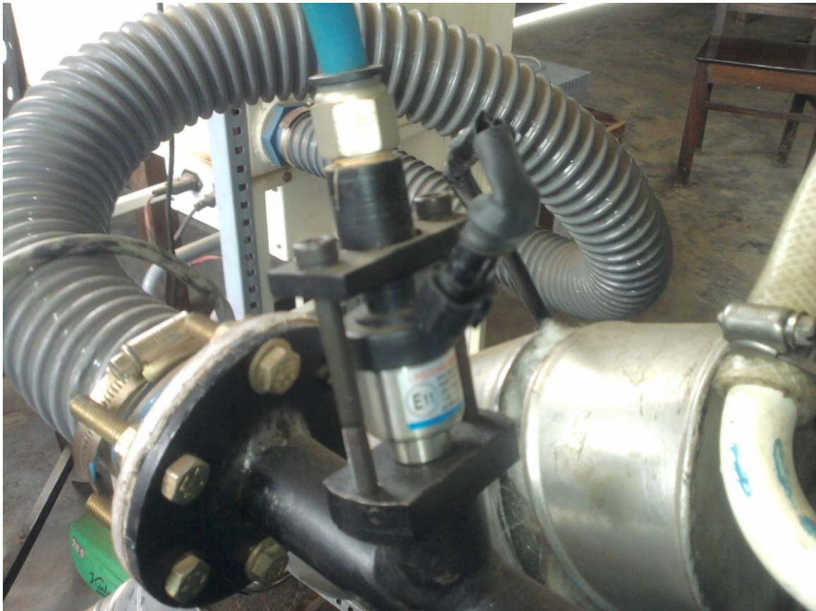
Figure 3. Photograph of biogas injection system
