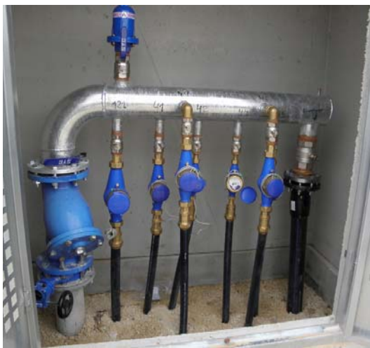
Figure 5. An example of a hydrant.
