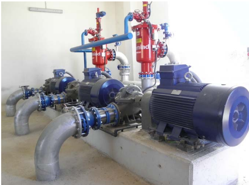
Figure 9. Examples of pumps.
